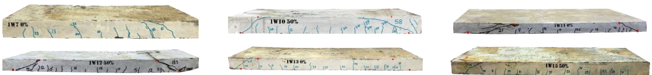
Fig. 8 Cracks pattern of slabs failed in shear.
